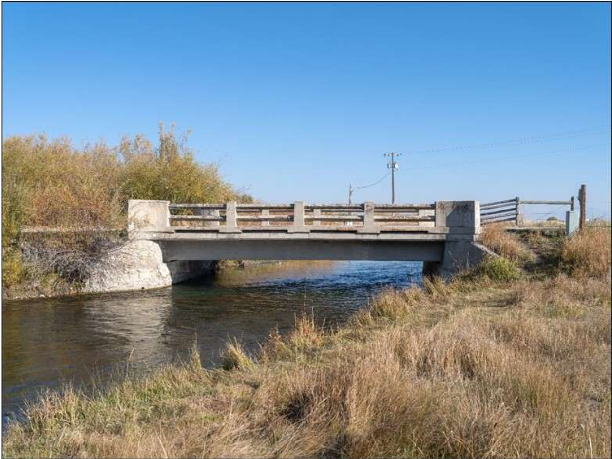
Poindexter Slough Fishing Access Bridge. North side. View to the south. MT_BeaverheadCounty_BridgesOfPoindexterSloughHistoricDistrict_0017.
