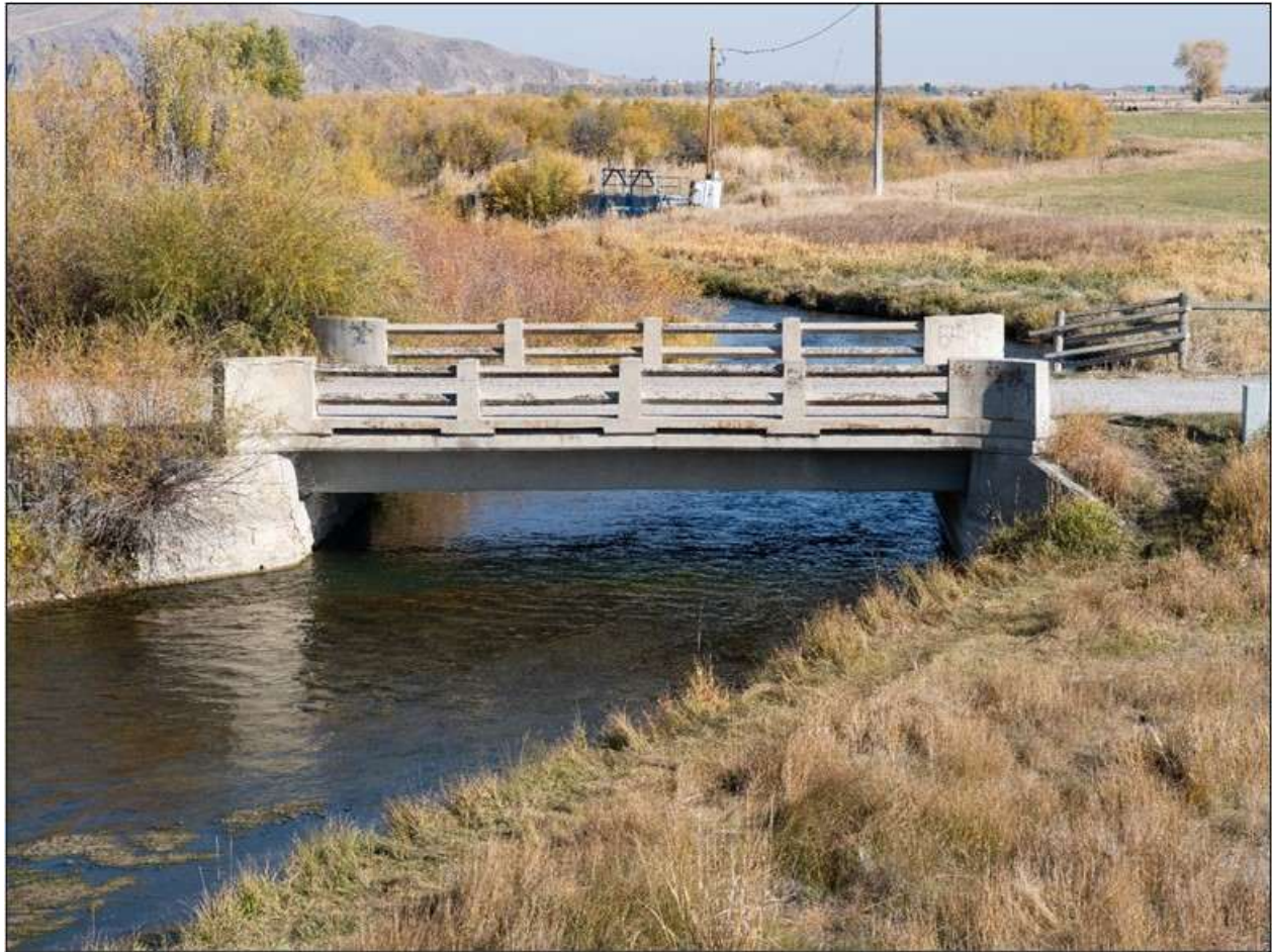
Poindexter Slough Fishing Access Bridge. South side. View to the north. MT_BeaverheadCounty_BridgesOfPoindexterSloughHistoricDistrict_0016.
