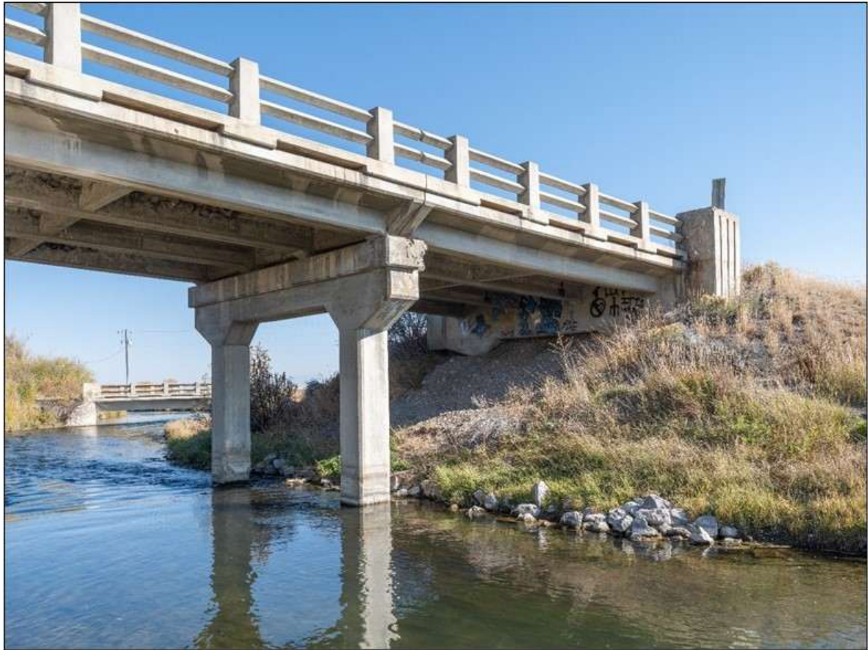
Poindexter Slough Bridge. Detail. Pier, underside, and guardrail. View to north. MT_BeaverheadCounty_BridgesOfPoindexterSloughHistoricDistrict_0008.
