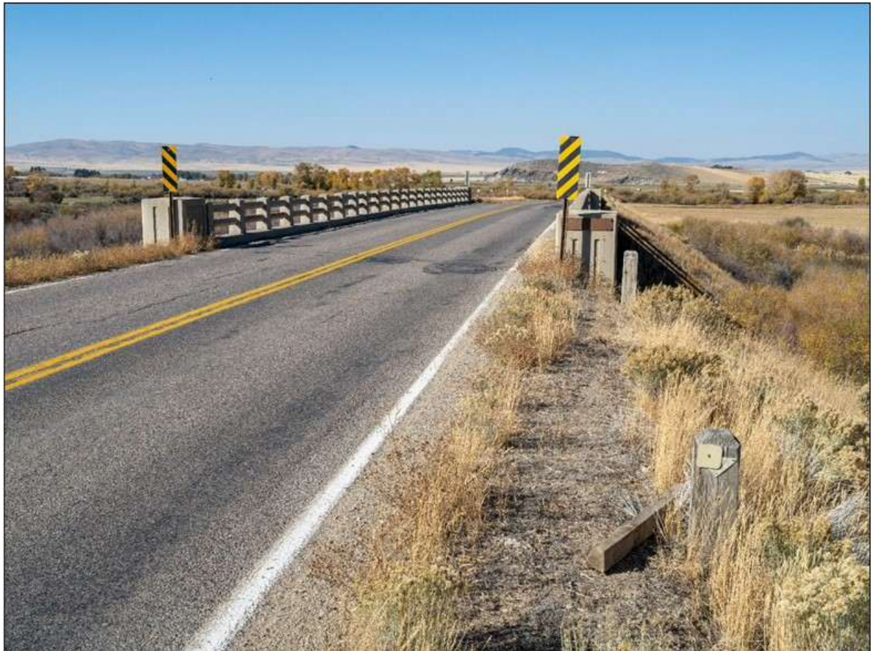
Montana Secondary 222/Old U.S. 91. Detail of guard posts. View to west. MT_BeaverheadCounty_BridgesOfPoindexterSloughHistoricDistrict_0023.
