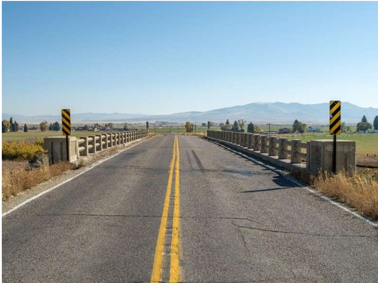
Montana Secondary 222/Old U.S. 91 and Poindexter Slough Bridge. View to east. MT_BeaverheadCounty_BridgesOfPoindexterSloughHistoricDistrict_0020.
