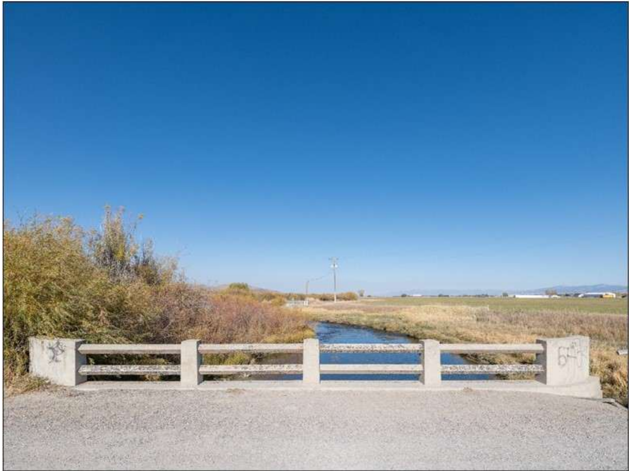
Poindexter Slough Fishing Access Bridge. Detail of north guardrail. View to the north. MT_BeaverheadCounty_BridgesOfPoindexterSloughHistoricDistrict_0018.
