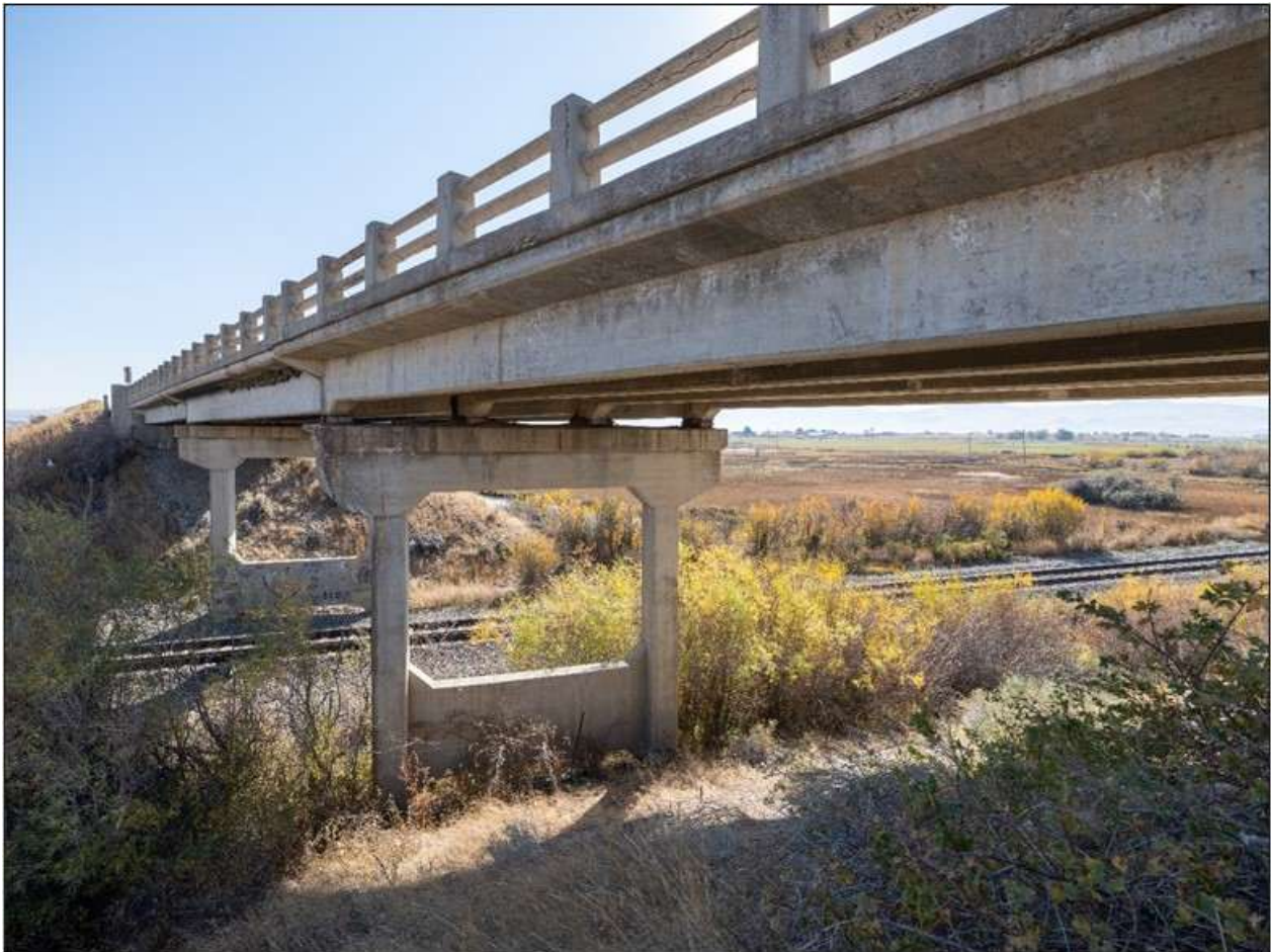
Oregon Short Line Overpass. Detail of bents and superstructure. View to the southeast. MT_BeaverheadCounty_BridgesOfPoindexterSloughHistoricDistrict_0014.
