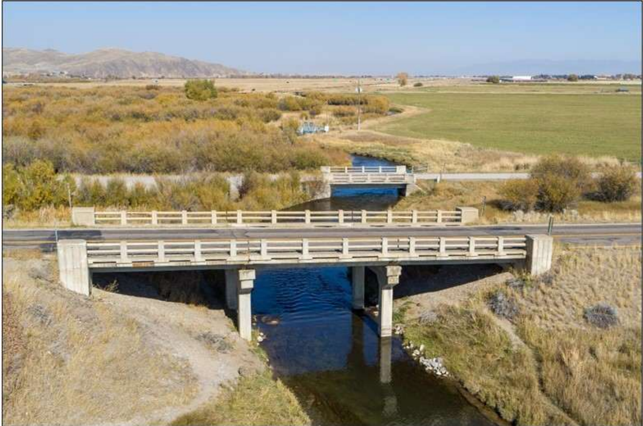
Poindexter Slough Bridge. South side. Poindexter Slough Fishing Access Bridge in background. View to north.
