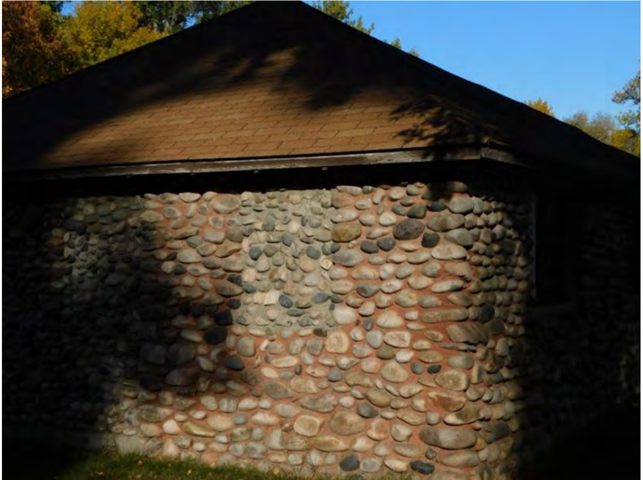
MT_YellowstoneCounty_RiversidePark_0019. Rifle Club building, looking east at filled in window from 1950s (notice mortar change after 1955). October 07, 2023.
